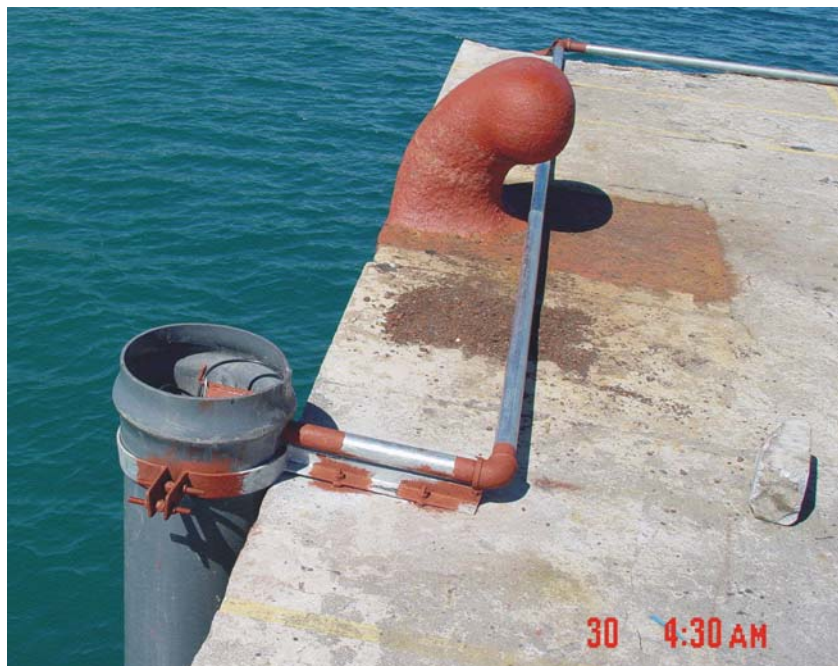
Stilling well, with pressure sensor
