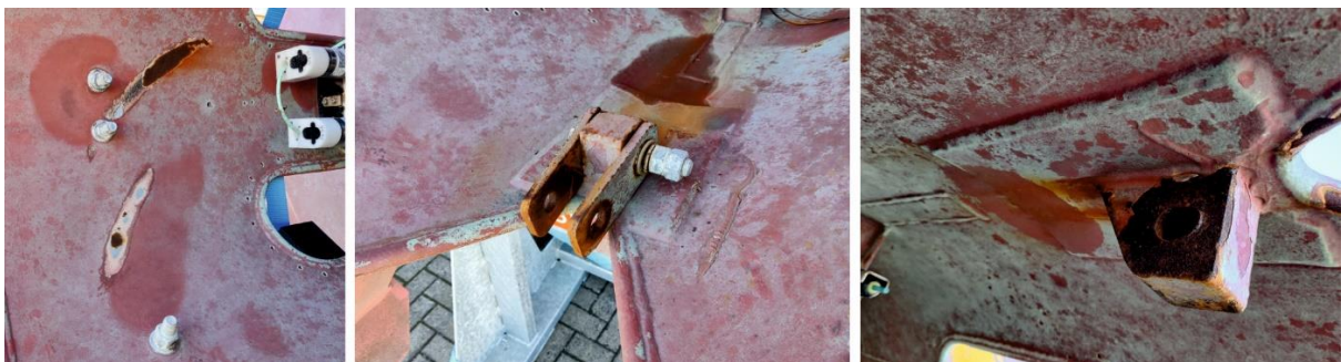
Figure 7.5: Damage inside the keel where the attachment bar became detached from the buoy
