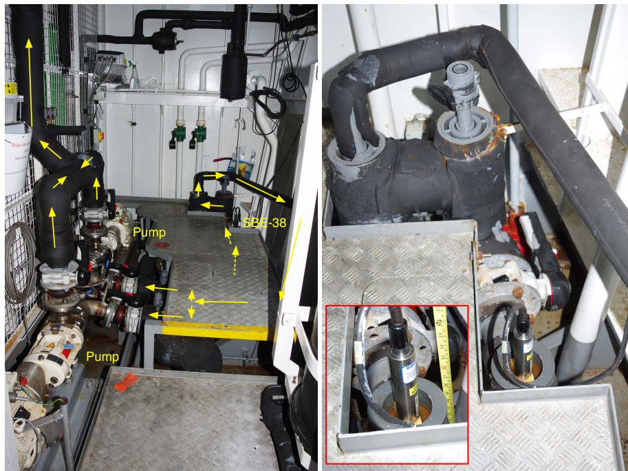
Figure 9.2: Pump room for clean seawater. Left shows the layout of the room with inlet + SBE-38 and pumps, right shows SBE-38 with inset showing the height of the instrument from the tank top (360 cm above hull baseline).
