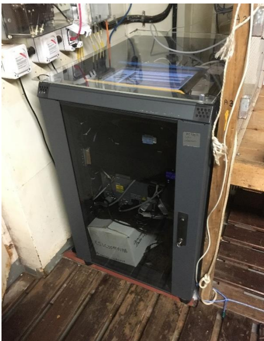
Figure 10.2: Mail room setup (right photo): Monitor (for the Dell PC and the Picarro internal PC) on the top shelf, Dell PC & UPS on the shelf below, and the Picarro on the lowest shelf (above two boxes of spares on the floor).
