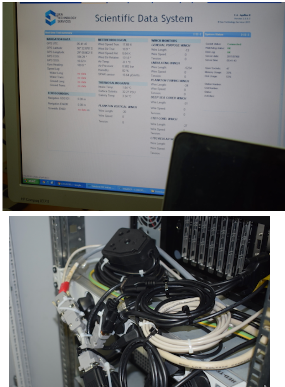
Figure 65 Top: issues with data transmission from echo sounder to the SDS. Bottom: Cables connecting the SDS system to the various sensors. The echo sounder is connected with the patched red-taped cables.
