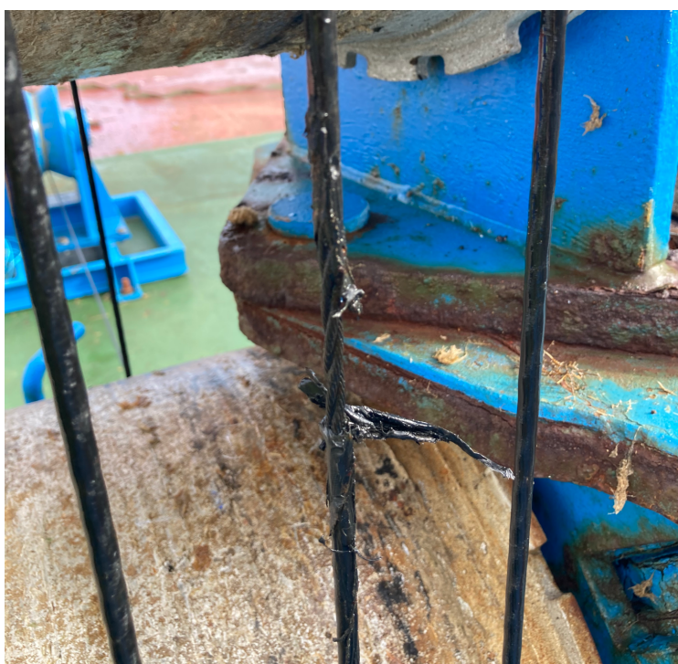
Figure 17.2 Showing shredding of the plastic jacket on the wire at WB2 around 200m.
