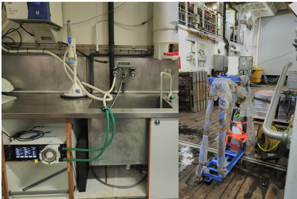
Figure 15.1 SubCTech system installed next to sink in Deck Lab, and its standard calibration gas cylinder in Hangar.
