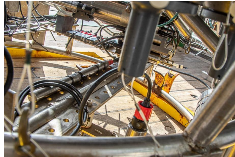
Figure 3.8: View of Xeos battery pack (left side of centre structure), Oceanids Hub (far structure under SBE-9plus) and ANB sensor to right of picture
