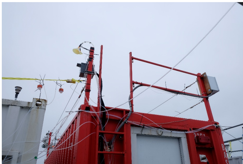
Figure 14. Photograph of the O 3 , NO x , SO 2 and CO inlets on the left (covered by the big and small funnel) and the NO y converter box on the right of the roof of the BAS container.
