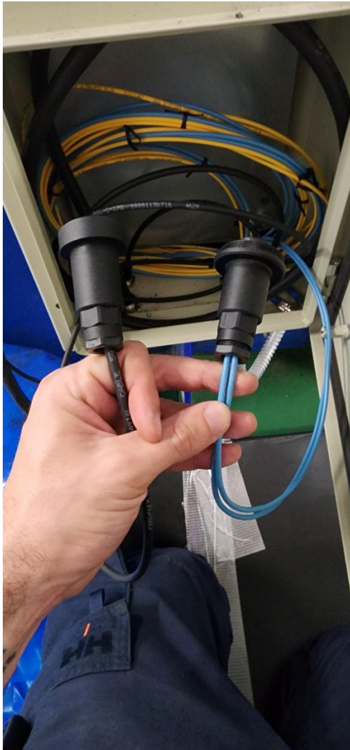
Figure 7.2-3. Wires mega tested inside the junction box on the CTD drum.
