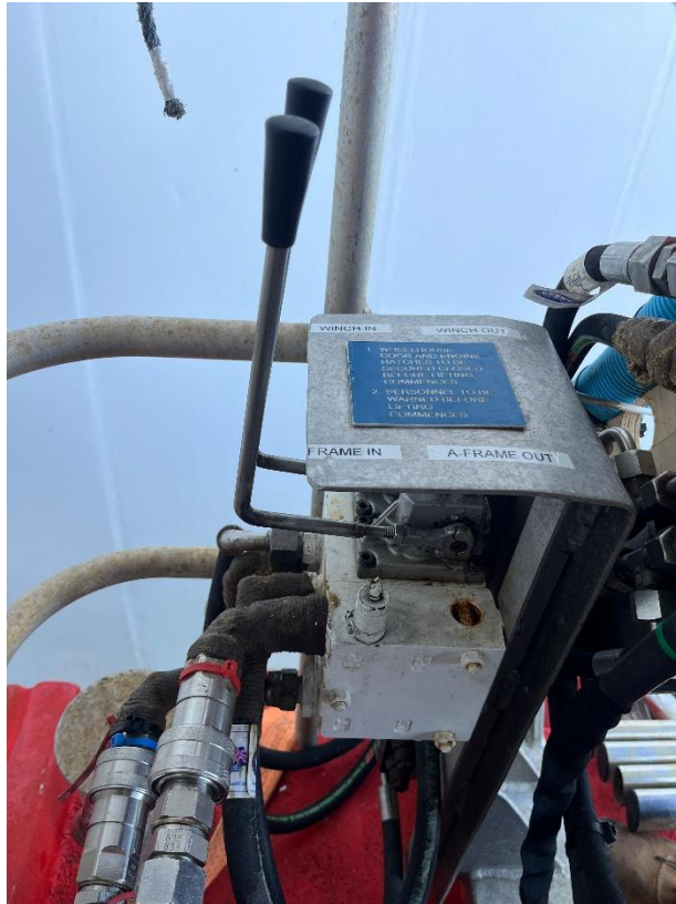
Figure 7.5-4. Raised A-Frame controls.
