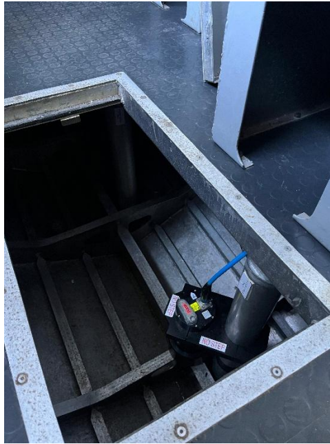
Figure 7.5-8. Cable pipes located inside Erebus haul.
